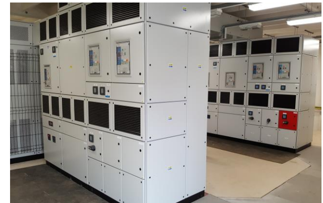
Switchboard room in Charnwood campus
