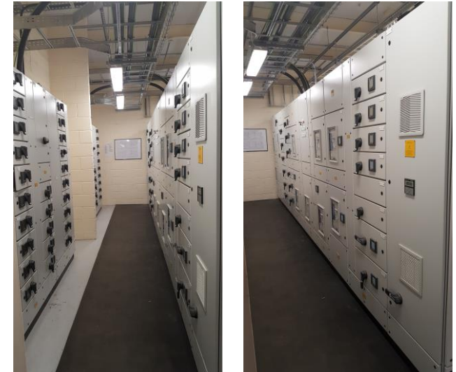
Switchboard room in Dewsbury Hospital
